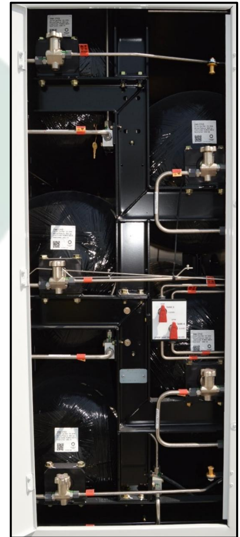
Back of Cab Access Door View (5 tank system)
